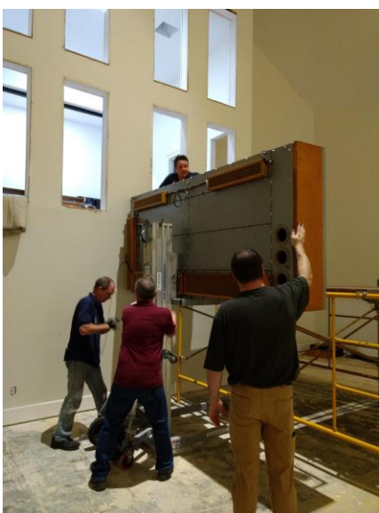
Installing windchest in the new organ room (Kevin, Jeff, Derek and Justin)
